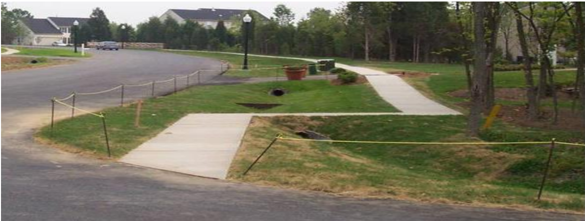
FIGURE 4-9 Recently Constructed Grassed Swale in Residential Area, Pembroke Woods Subdivision in Emmittsburg, MD (Courtesy of Mike Clar, Ecosite, Inc., Columbia, MD)
